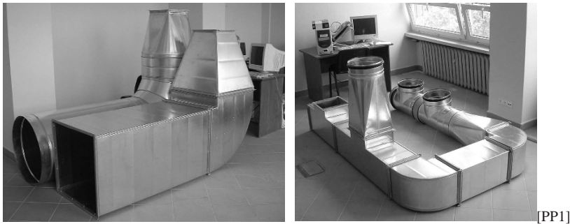
Fig.5. Ventilation ducts used as test stage
