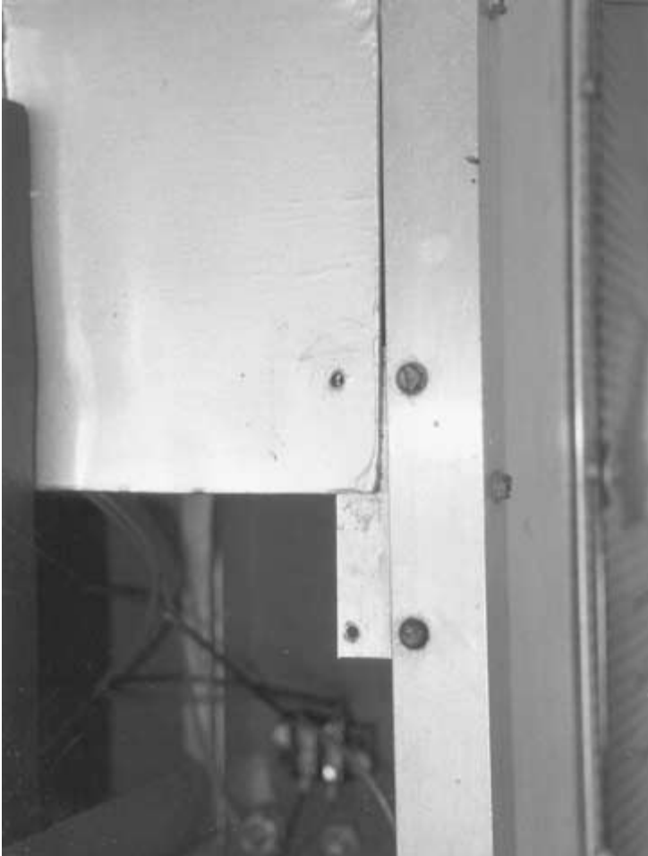
FIGURE 6-7. Hole in both access panel and mounting tab.
