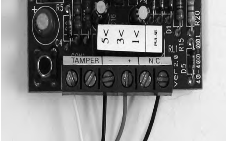
Figure 6-16. Simplified power and sensor connections made possible with EOL resistors pre-soldered under the PCB
