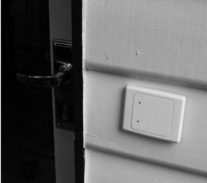
Figure 14-17. Reader mounted inside a wall plate fitted beside a door
