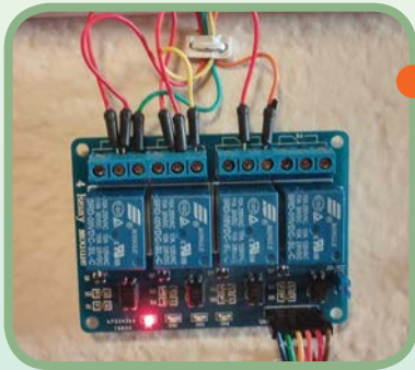
The SainSmart relay is wired between the Raspberry Pi and the HVAC control unit
