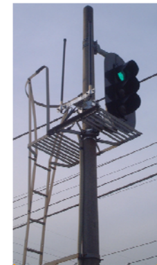
Wayside WLAN Bridge
