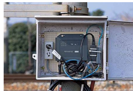
Wayside WLAN Antenna
